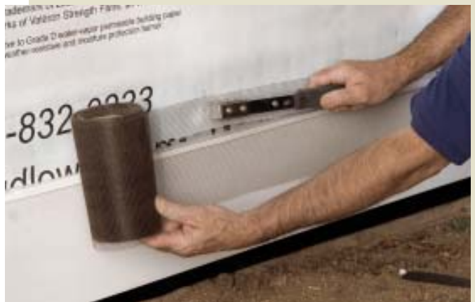
Figure 5. Two 3-inch-wide polypropylene-mesh vent strips — one at the top, one at the bottom — help provide continuous ventilation behind the siding (top and center). For good measure against bugs, the strips were wrapped in insect screening, installed first (above).
